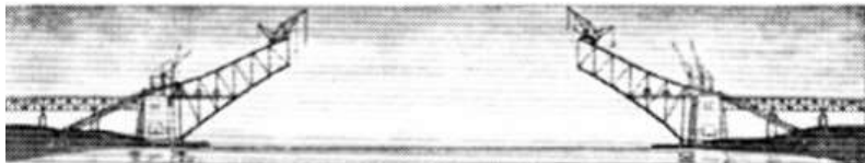
(c) Six panels on each side erected; creeper cranes continue to advance as work progresses
